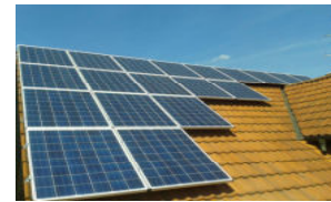
9,4 kWp Photovoltaik-Mieter-Strom Wolfersdorf, 2015
